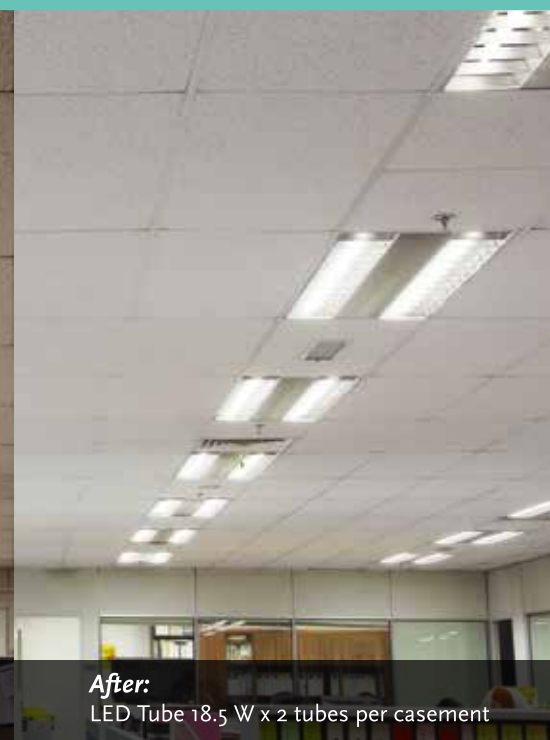
Before: Fluorescent 36 W x 3 tubes per casement
